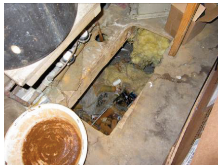
Hole in Mechanical Room Floor
