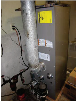
Installed Lennox Furnace
